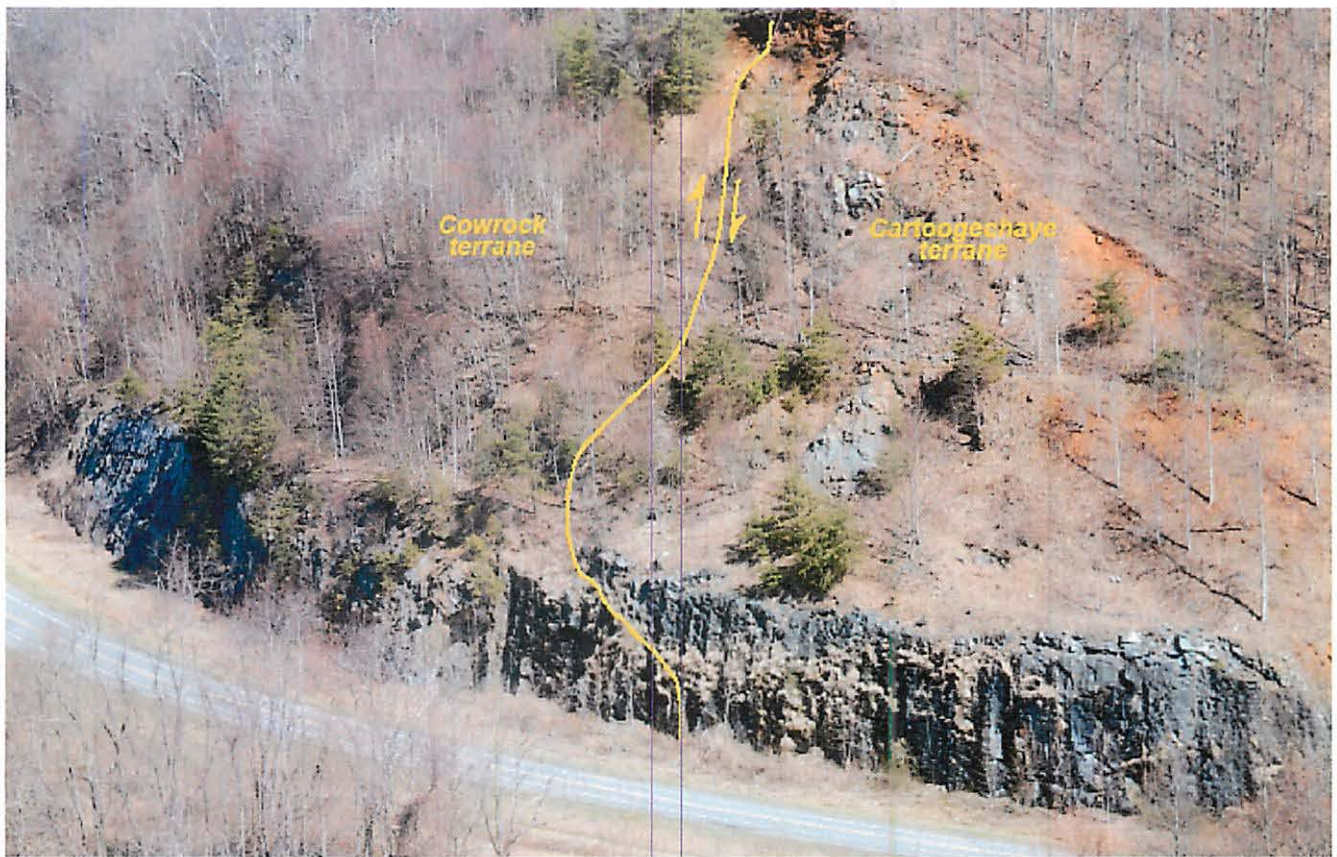
Figure 12. Oblique aerial photograph of Stop 9A with the trace of the Chunky Gal Mountain fault shown.
